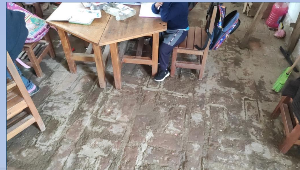
The floors of all classrooms are damaged.
