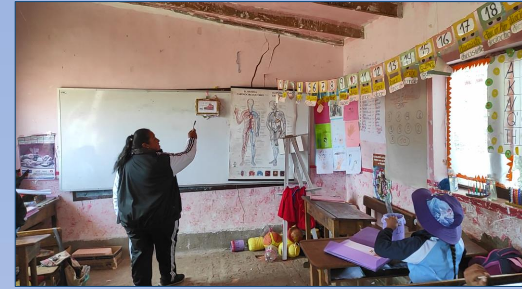
Damaged wall with cracks in one of the current classrooms and there is also a leak in the roof.
