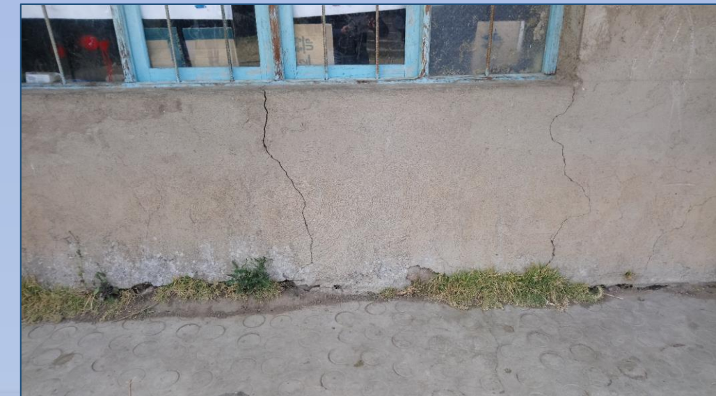
Externally the classrooms are very deteriorated and all have cracks.
